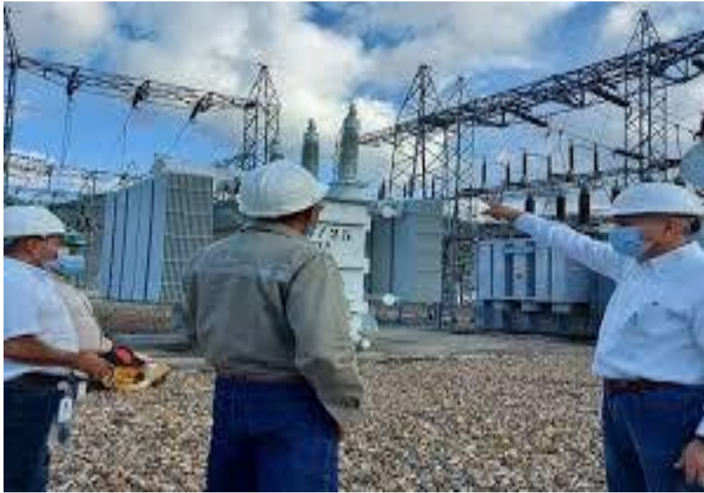
Figure 67. Tibú Substation – Cesar
